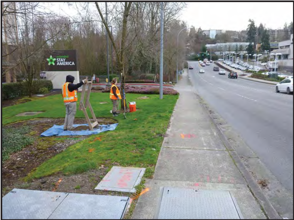
Figure 23. Shovel test excavations on NE Main Street in Zone 81 A3, view to the east. Note locations of buried utility lines denoted with orange spray paint.
