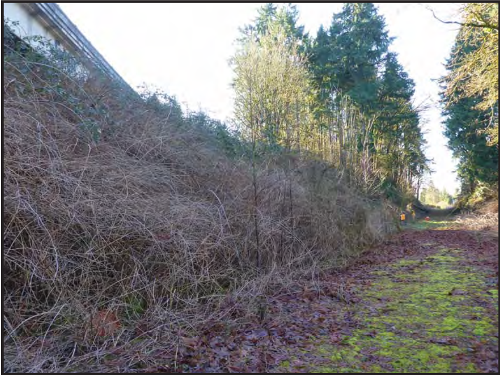
Figure 6. Photograph showing a cut slope covered by impenetrable blackberry bushes, view to the south-southeast.
