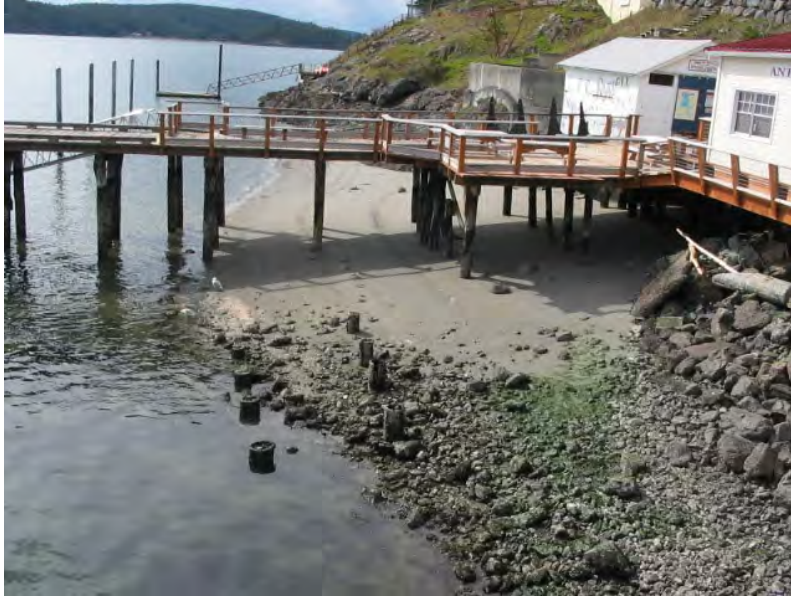
Figure OR-3 Shoreline Area to the West of the Orcas Island Ferry Terminal
