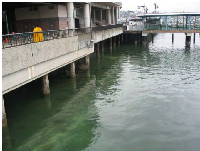
Figure BR-4 Shoreline Area to the East of the Bremerton Ferry Terminal
