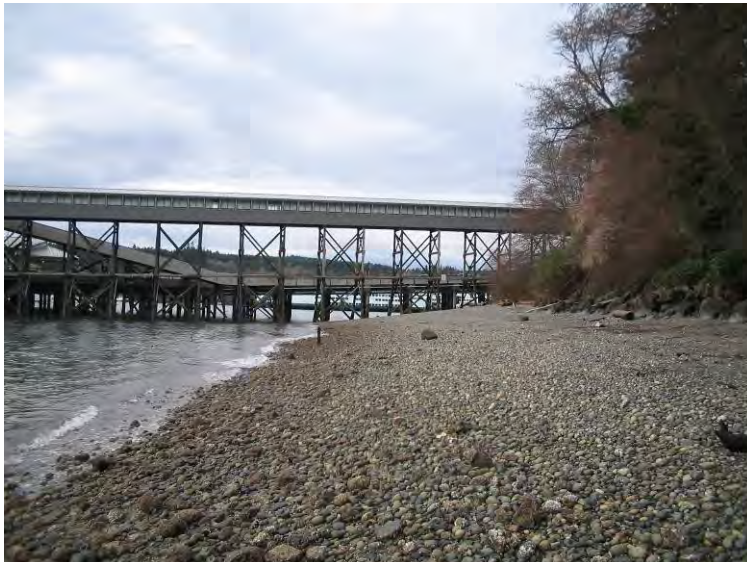
Figure BA-4 Beach Area on North Side of Bainbridge Island Ferry Terminal
