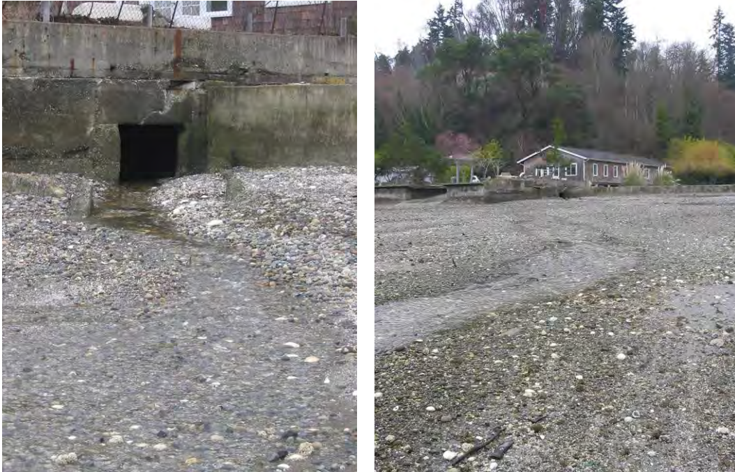
Figure TA-5 Concrete Culvert Carrying Talequah Creek and the Creek as it Flows onto the Beach
