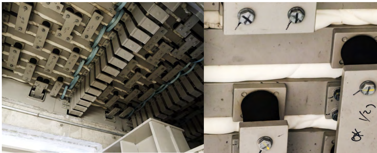
Figure 4-4. Underside of the MEJ with viscoelastic foam strips stuffed into the gaps.
